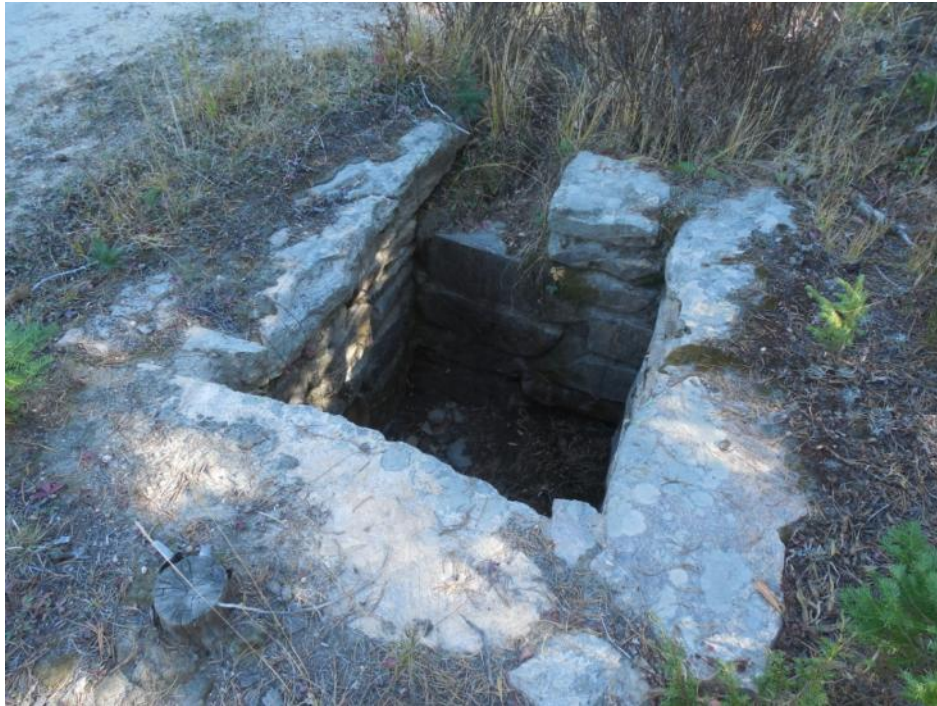
One of the many catch-basins long the Deadman Road built by the CCC.
